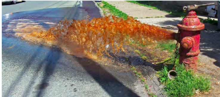
Figure 5-7 "Fire Hydrant Flushing Rusty Water," Photo by Daniel Case
