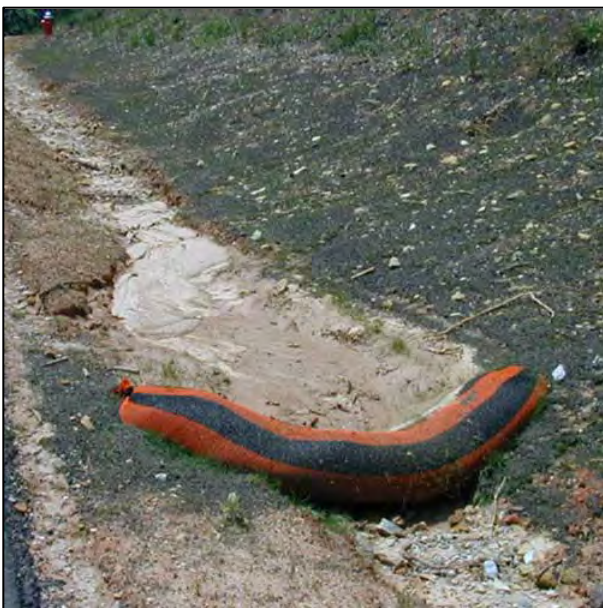
Sediment Tube used in a Ditch Setting
