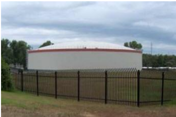
Figure 34. This equalization basin was installed to store sewer during times of peak flow and when sewer capacity is at a maximum.
