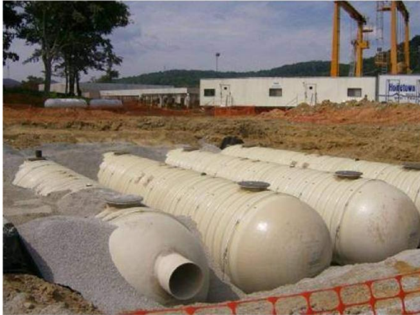
Figure 10.4. Example of Multiple Fiberglass Cisterns in Series (Source: VADCR, 2011)
