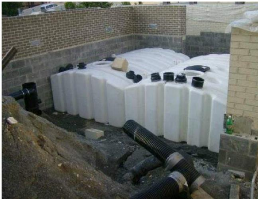
Figure 10.5. Example of two Polyethylene Cisterns (Source: VADCR, 2011)
