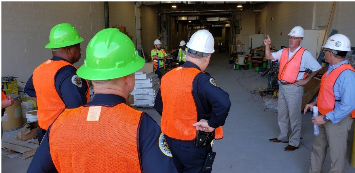
Officers will enter the new Downtown Detention Center through a garage at Gay Street and 2 nd Avenue North.
