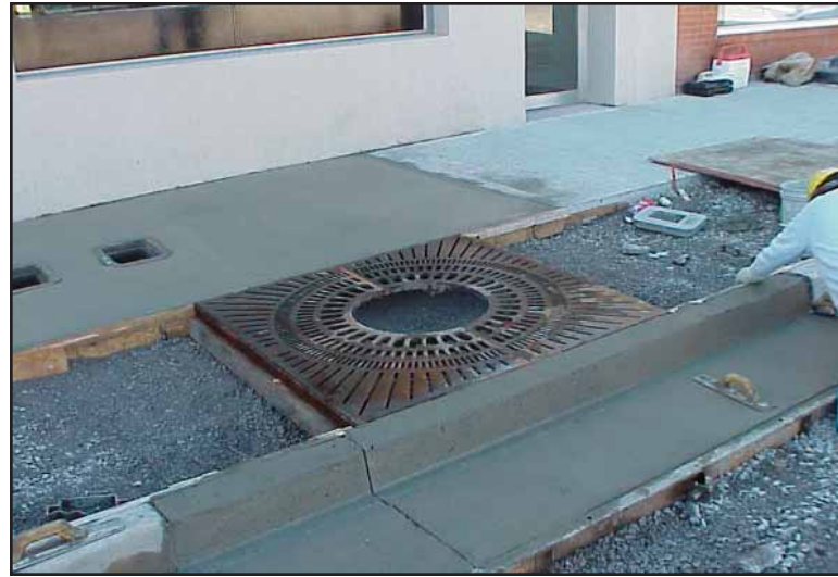
Photo 8.4—The photo and diagram to the right (Figure 14.1) both show the correct installation of a tree grate with structural soil. Urban trees are especially vulnerable to the stress created by their environments. In order to help ensure their survival, special considerations must be given to the size and types of areas in which they are planted. Photo above for installation demonstration only; preferred tree grate appears below.
