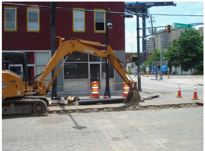
Figure 8. Atlanta Streetcar Project construction at 252 Auburn Avenue, NE. Note how access to Auburn Avenue businesses is obstructed.
