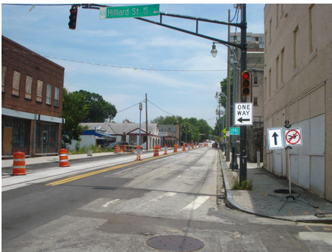
Figure 3. Hilliard Street @ Auburn Avenue looking east. Note that the a significant portion of the street is closed due to construction of the Atlanta Streetcar Project.
