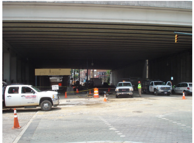
Figure 10. Atlanta Streetcar Project construction on Auburn Avenue at underpass beneath I-75/I-85. This feature is somewhat similar to the I-40 underpass on Jefferson Street except for the fact that no aesthetic improvements have been made at the Auburn Avenue site. The underpass is used for community events such as the Atlanta Caribbean Carnival - http://www.atlantacarnival.org/main.html
