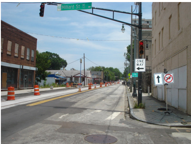
Figure 3. Hilliard Street @ Auburn Avenue looking east. Note that a significant portion of the street is closed due to construction of the Atlanta Streetcar Project.
