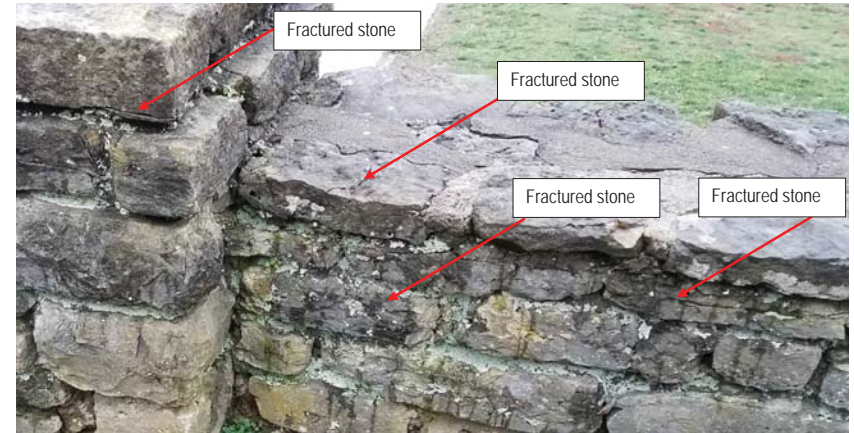
Photo 3 - Example of cracked and fractured stones.
