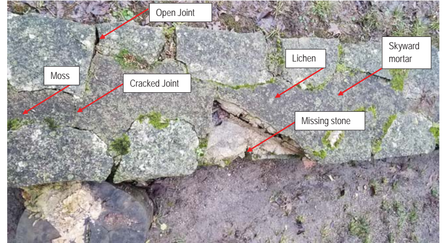
Photo 12 - The top of the wall with skyward facing mortar, cracks, open joints, moss and lichen.
