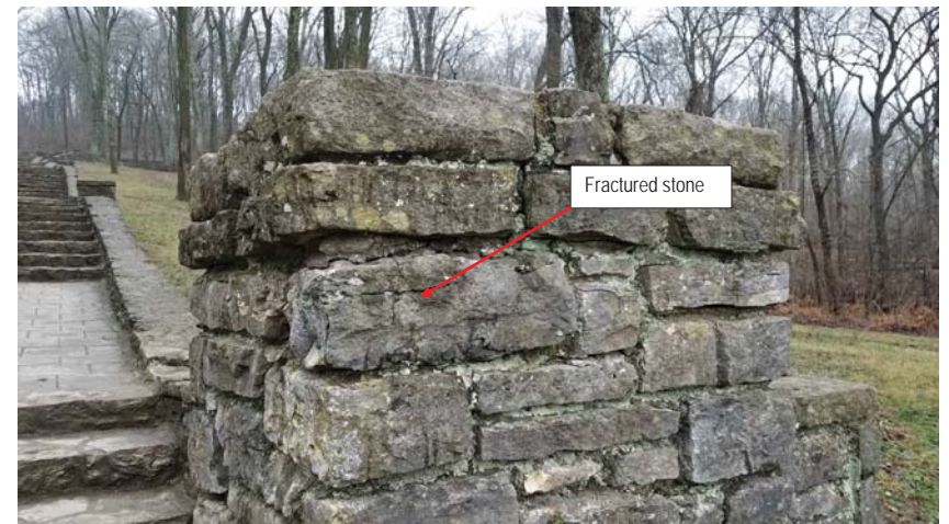
Photo 4 - Example of cracked and fractured stones.
