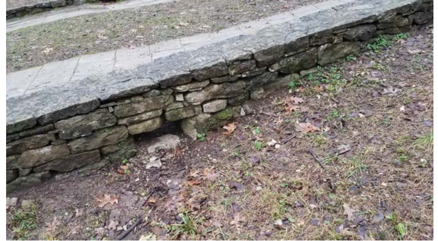
Photo 23 - Sidewall where all mortar has washed out and required rebuilding. Moisture from lawn side of wall back washing into scupper due to slopes.
