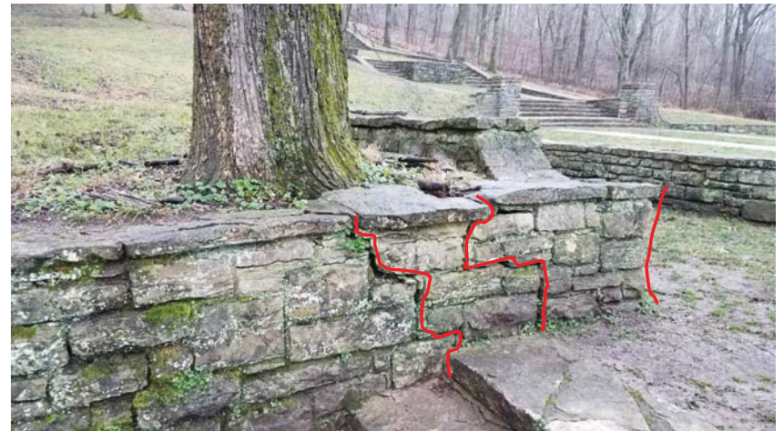
Photo 16 Displacement of wall due to tree roots. This portion of the wall needs to be reset.
