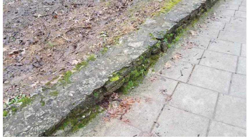
Photo 19 – Low retaining wall to be rebuilt. All mortar has washed out, wall is displacing. Note wash out of soil in lawn adjacent. Water mitigation must be completed before masonry work.
