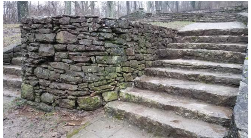
Photo 20 - Retaining wall to be rebuilt. All mortar has washed out, wall is displacing. Note irregular height of treads and lack of handrails and guard rails.
