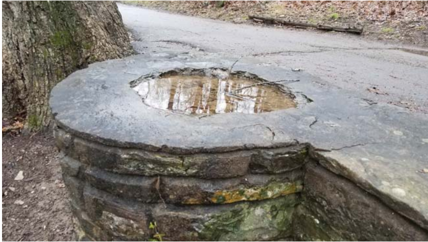
Photo 6 - Example of skyward surface in need of stonework or mortar wash to prevent water accumulation.
