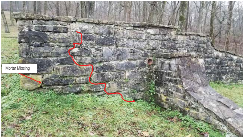
Photo 14 Cracking through wall due to minor differential movement; Crack to be cut out and repointed
