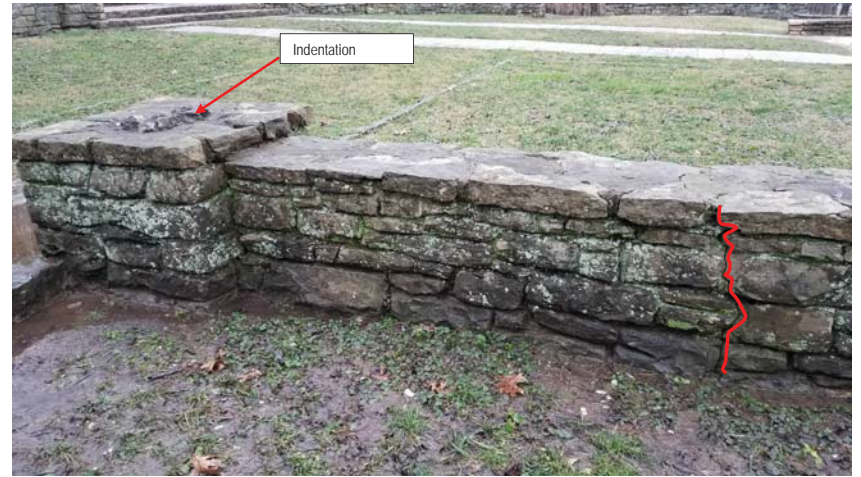
Photo 15 - Wall with differential movement causing crack; Crack to be cut out and repointed. Indentation in top of pier catching water and in need to filling with stone or mortar wash
