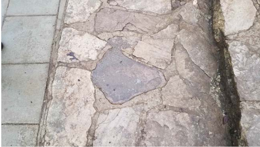
Photo 5 - Example of skyward surface in need of mortar wash to prevent water accumulation.
