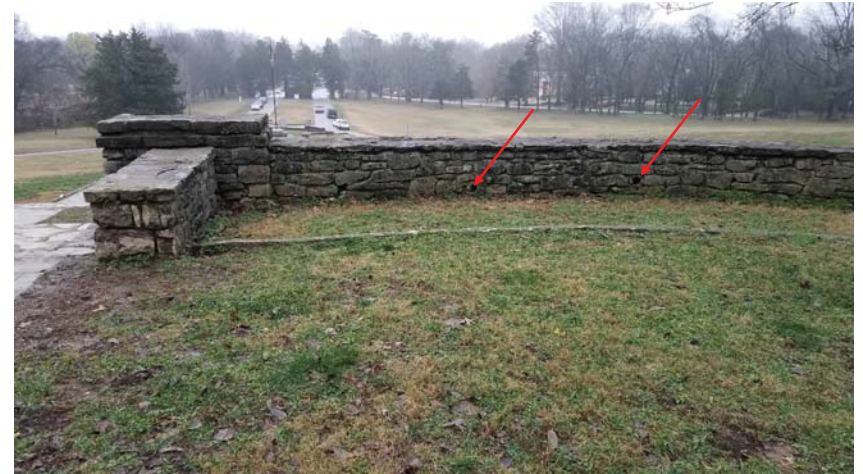
Photo 8 - Retaining wall where original clay drainage pipes have ended up well above grade level, rendering them ineffective.
