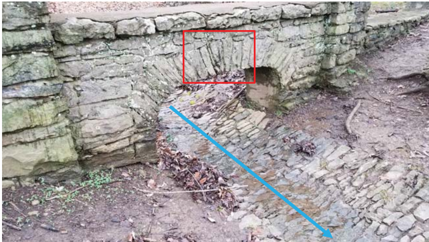
Photo 35 - World War I Memorial front of bridge with area of concern marked (see next photo)
