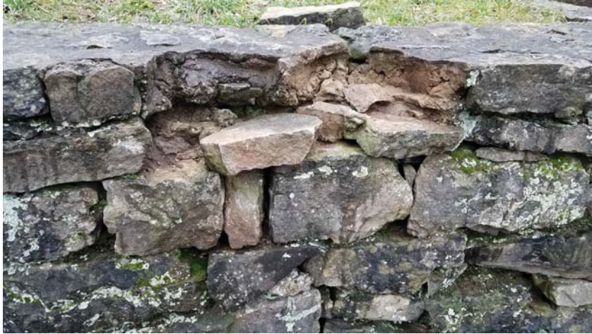
Photo 21 - Retaining wall to be rebuilt. All mortar has washed out, wall is displacing.
