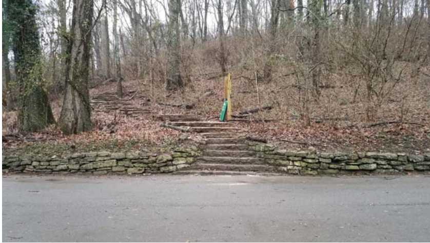
Photo 25 - Retaining wall at south side of roadway at top of stairs was dry stacked and has displaced. Proposal to reset wall with mortar.
