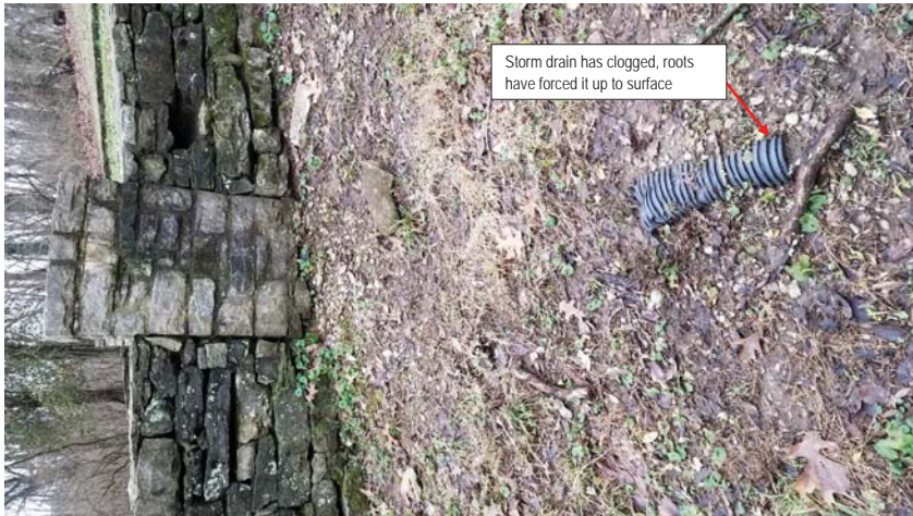
Photo 22 - Storm drainage placed to west of previous photo has failed.
