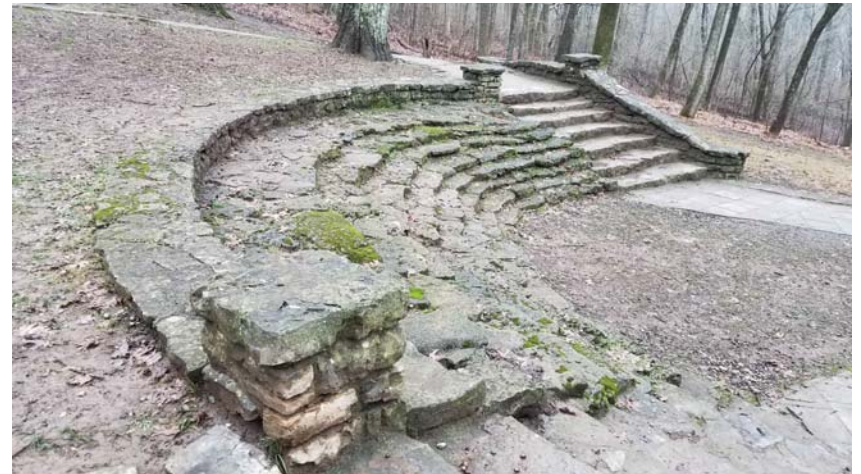
Photo 24 - Crescent area of steps / seating that has displaced and is washing out due to saturation from surface groundwater
