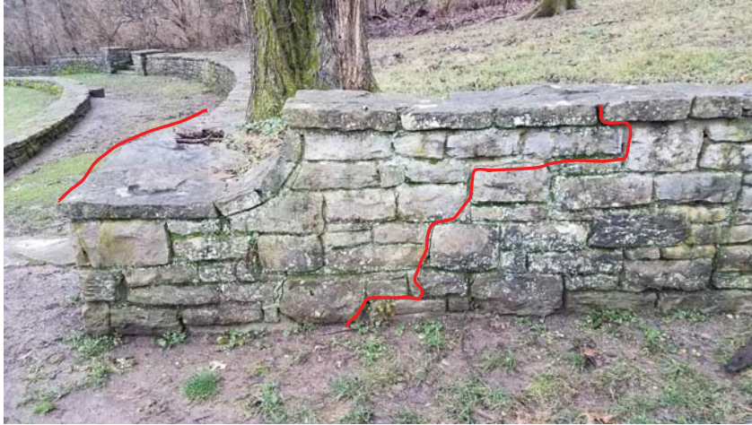
Photo 17 Displacement of wall due to tree roots. This portion of the wall needs to be reset.
