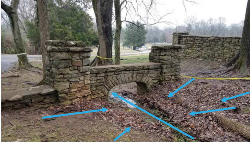
Photo 34 - World War I Memorial back of bridge, with path of water from south, moving east - quantity of water in the recent storm event resulted in overwhelming the storm drainage, and deposition of debris.
