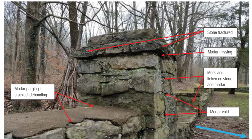
Photo 37 - World War I Memorial west side of bridge. Note spalling stones, poor condition of mortar, typical of the memorial.
