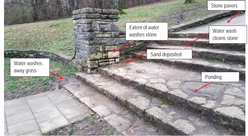
Photo 7 - Area of steps where water washes down, deteriorates mortar, deposits sand and mud, and saturates masonry causing heavy moss growth.
