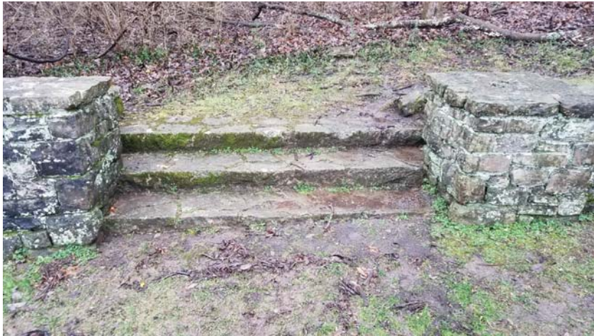
Photo 10 – Steps are comprised of individual stones, in a flagstone pattern, with inconsistent tread depth and riser height, with wide mortar joints skyward facing. Note lack of handrail.
