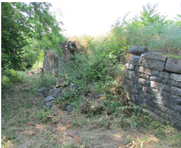
Figure 61. Collapse area at East Bastion retaining wall — reinforced earth retrofit (1200AE, 2013).
