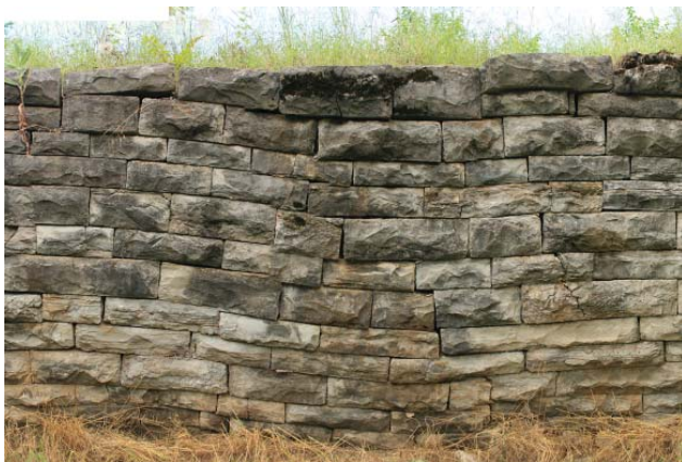
Figure 76. Sagging wall, possibly due to poor soils, animal burrows, or undermining (JMA, 2013).
