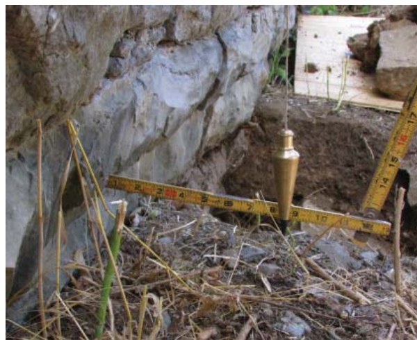
Figures 58a and 58b. Wall profile survey method with masons rule and plumb-bob (plummet) at horizontal joints at top, middle, and bottom of wall (1200AE, 2013).
