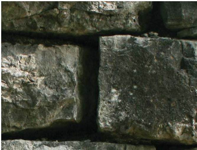
Figure 80. Open head joints (JMA, 2013).
