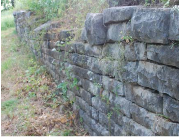
Figure 74. Localized wall displacement and missing capstones (JMA, 2013).
