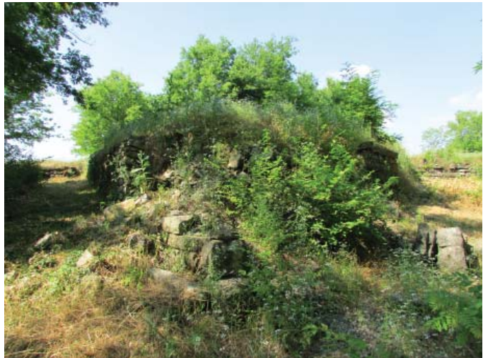
Figure 63. Collapse area at Redan No. 7 retaining wall (1200AE, 2013).
