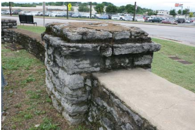
Figure 100. End pier of original wing wall extending from south end of gateway (JMA, 2013).
