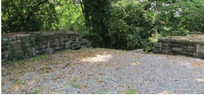
Figure 111. Collapse at southwest corner of wall (1200AE, 2013).
