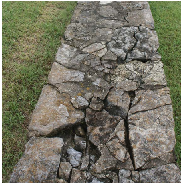
Figure 104. Water infiltration damage due to cracked or missing mortar joints at top of a portion of northwest wing wall of entrance gate structure (JMA, 2013).
