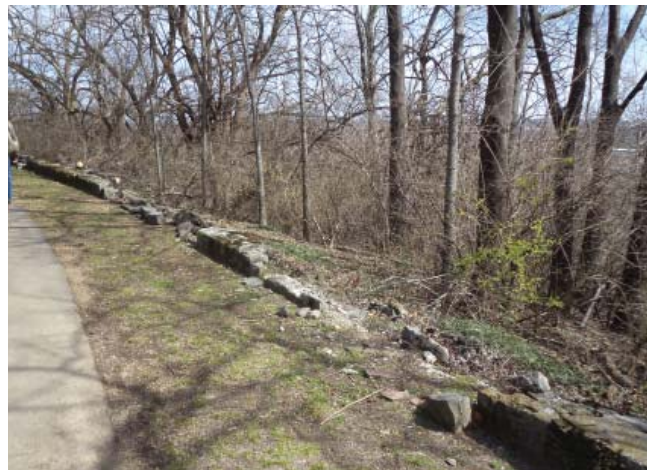
Figure 109. Damaged section of loop road retaining wall (JMA, 2013).
