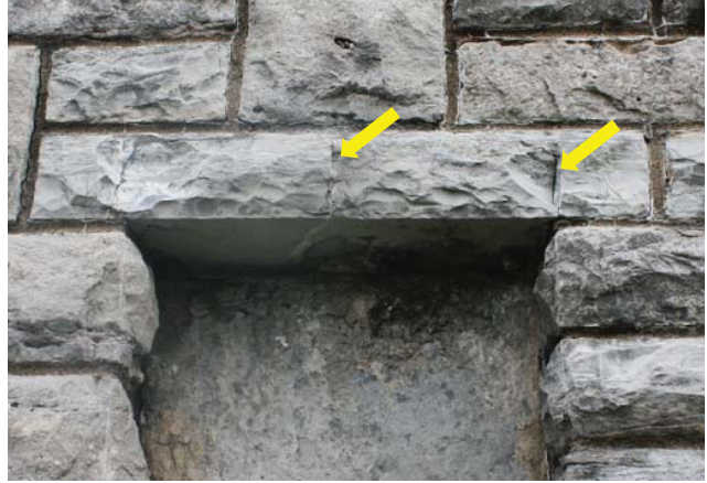
Figure 96. Lintel over niche in north-central pylon at entrance gate cracked in two places, giving appearance that limestone inset is holding lintel in place (JMA, 2013).
