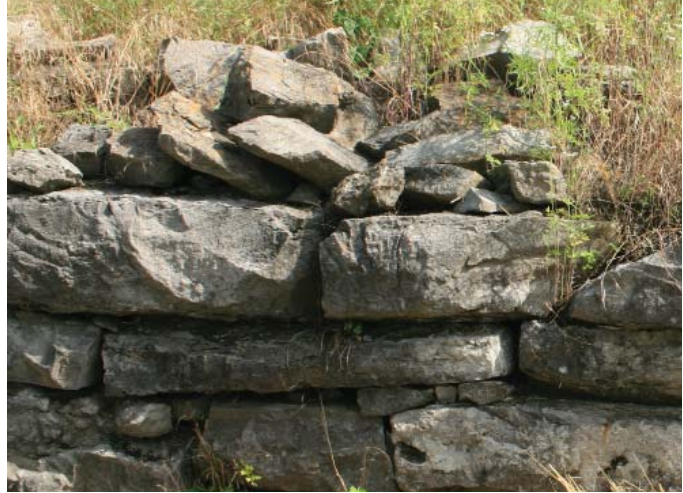
Figure 77. Stone rubble piled on top of wall (JMA, 2013).
