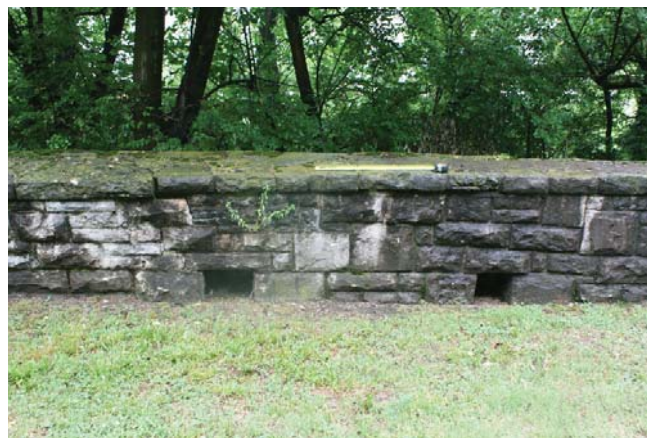
Figure 110. Drainage outlets built into the parapet. To the left, the wall is sagging due to structural instability (JMA, 2013).
