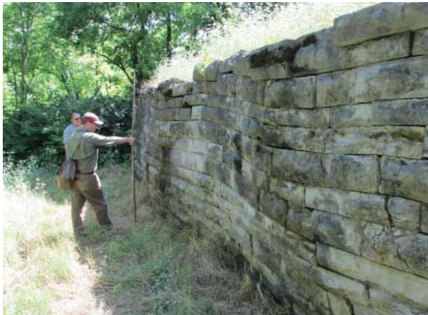
Figure 60. Bulging and out-of-plane rotation along east elevation of West Bastion (center and left), vertical cracking of stones to right, and dislodged and lost capstones (1200AE, 2013).
