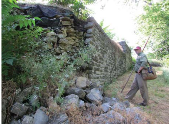
Figure 62. Collapse area at East Bastion retaining wall — reinforced earth retrofit (1200AE, 2013).
