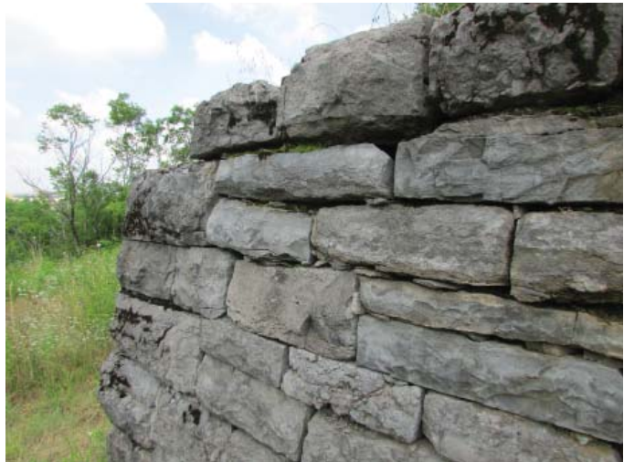
Figure 66. Various stages of delamination in exterior facing stones (1200AE, 2013).
