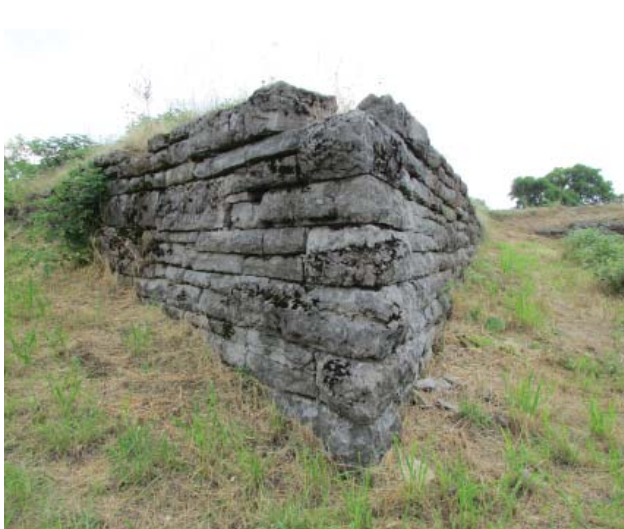
Figure 70. Loss of capstone units and delamination of exterior surface of stones (1200AE, 2013).
