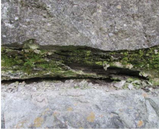
Figure 68. Initial stages of delamination and exfoliation in exterior stones (1200AE, 2013).
