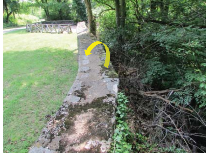
Figure 114. Rotation of parapet towards the interior (1200AE, 2013).
