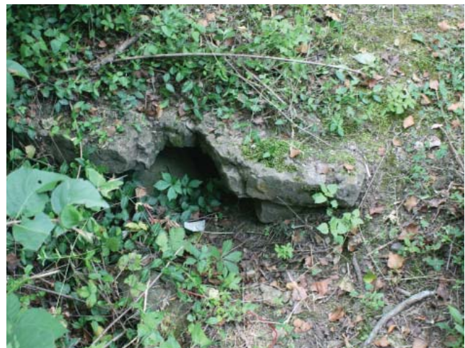
Figure 116. Partially-buried limestone drop inlet cover (JMA, 2013).
