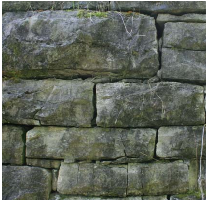
Figure 78. Large stones laid in top half of wall alter the center of gravity, promoting wall overturning and crushing stones in wall below (JMA, 2013).
