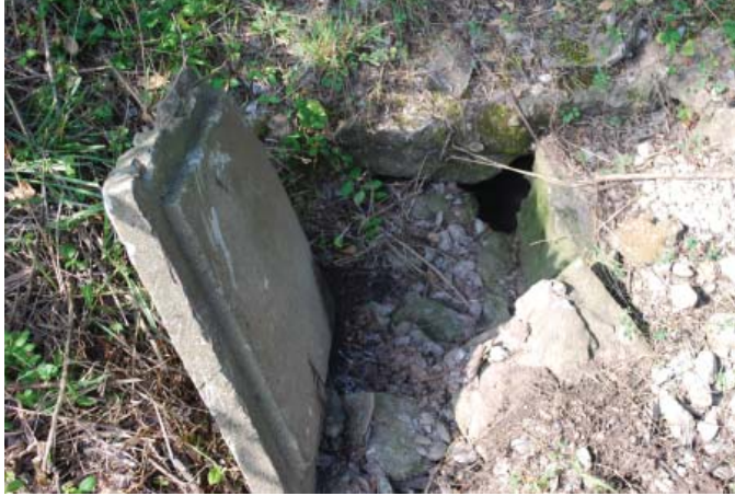
Figure 117. WPA drainage inlet: stone cover replaced with precast concrete cap and culvert filled with sediment and debris (JMA, 2013).
