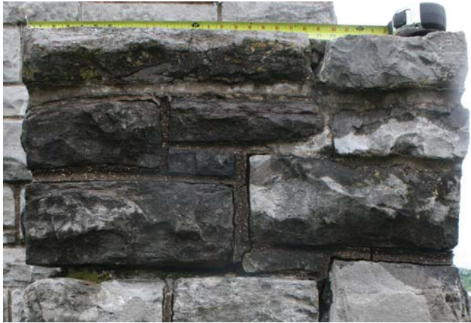
Figure 93. Entrance gate pier exhibits hairline-to-minor cracking in mortar joints, some open joints, and inappropriate repair in joint below cap (JMA, 2013).
