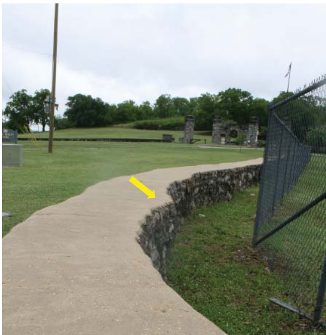
Figure 101. Bowing and displacement of southern wing wall, rear view (JMA, 2013).
