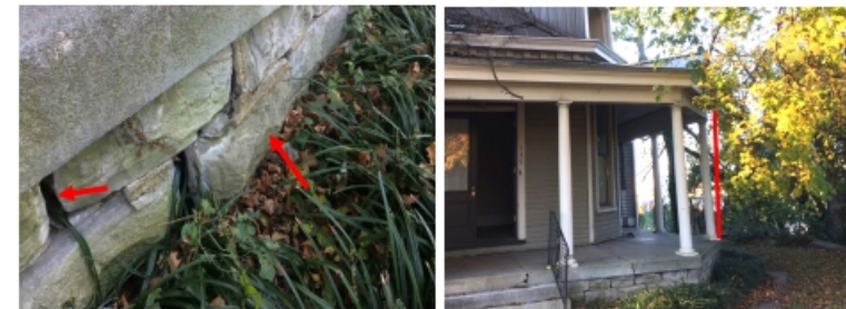
22. The porch section at the front door is cracked in the center and sloping towards the left, directing any water that blows onto the porch surface towards the right side wall of the front living room.
