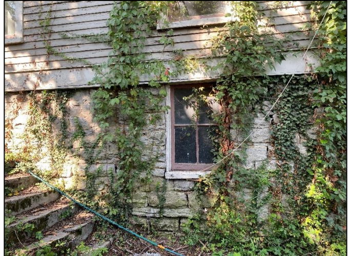
Figure 7: Foundation wall on the east side shows mortar joints that have deteriorated but is overall in good condition.
