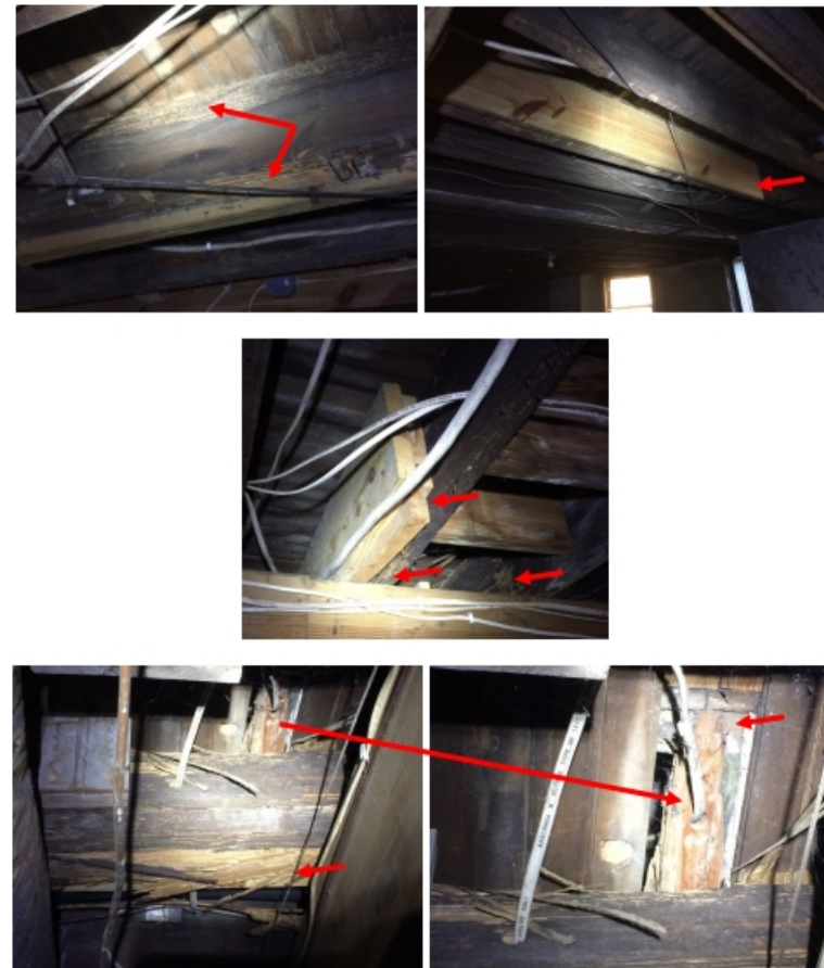
Undermined wall framing due to insect damaged floor
