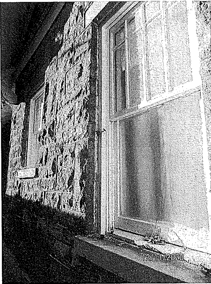
Photograph 21: Wall movement (left side) at window casement.
