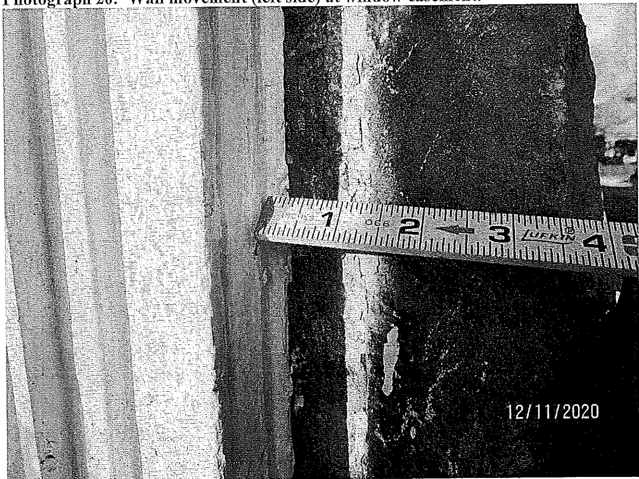
Photograph 20: Wall movement (left side) at window casement.
