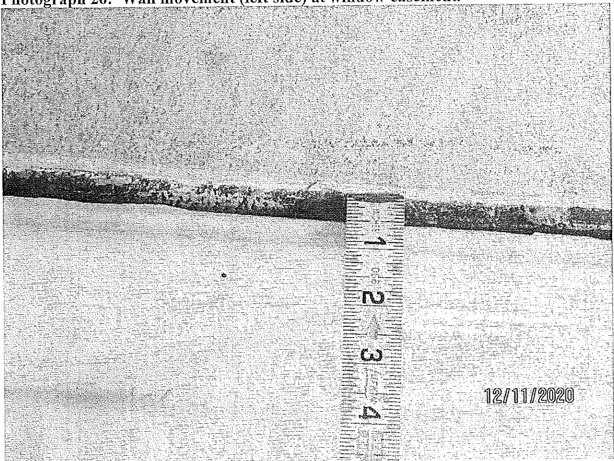
Photograph 26: Wall movement (left side) at window casement.
