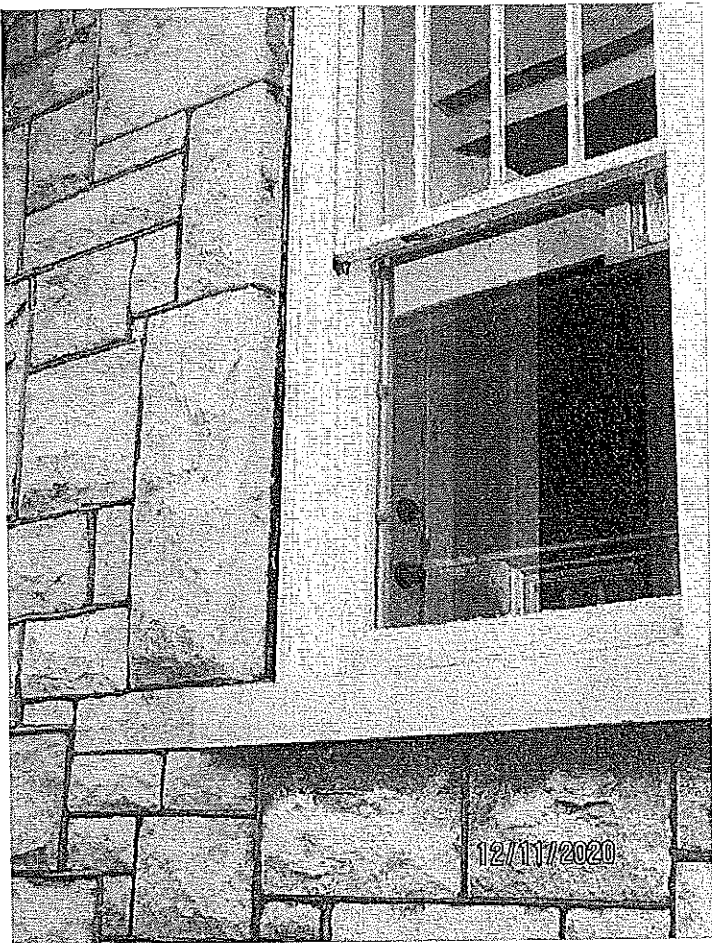
Photograph 13: Wall movement (right side) at window casement.
