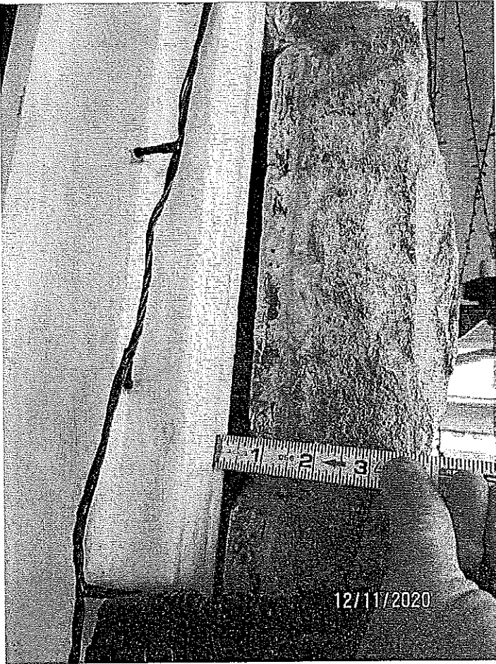
Photograph 3: Wall movement at front wall at doorway.
