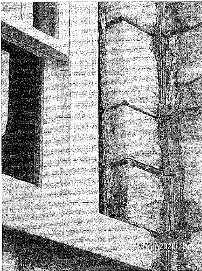
Photograph 7: Wall movement (right side) at window casement.
