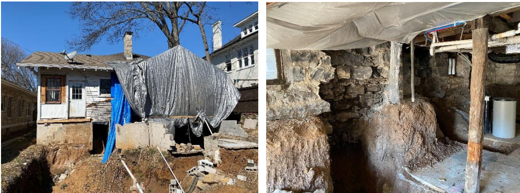
Figures 3 and 4: Rear façade and interior view, as seen on February 25, 2021, after receipt of the demolition application.
