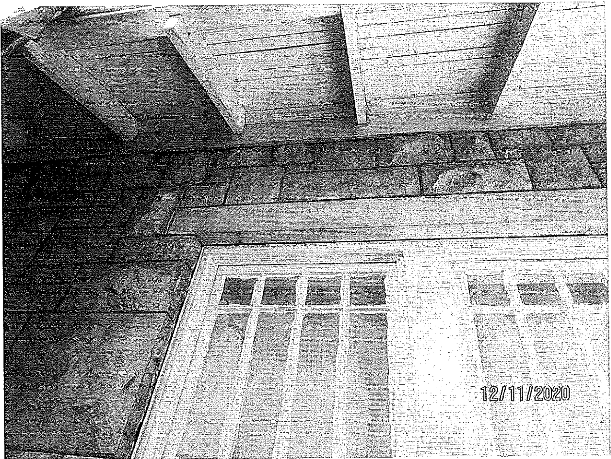
Photograph 25: Wall movement (left side) at window casement.
