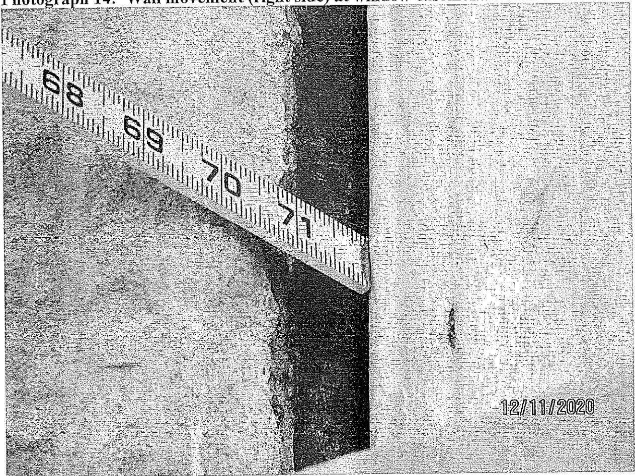
Photograph 14: Wall movement (right side) at window casement.
