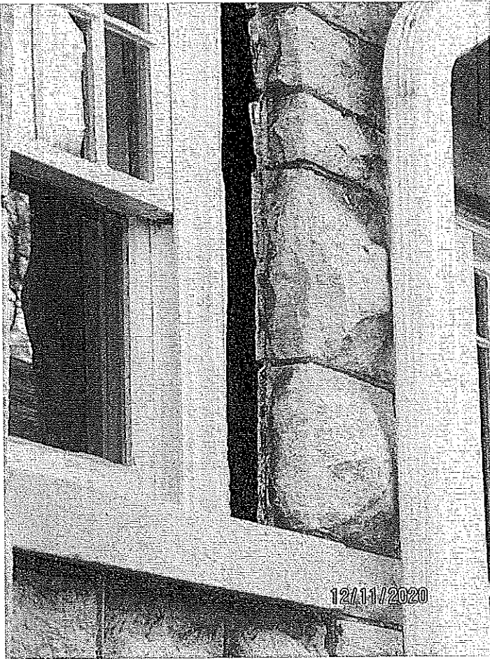
Photograph 9: Wall movement (right side) at window casement.
