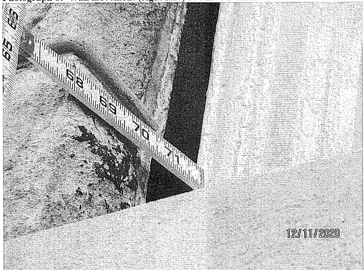
Photograph 8: Wall movement (right side) at window casement.
