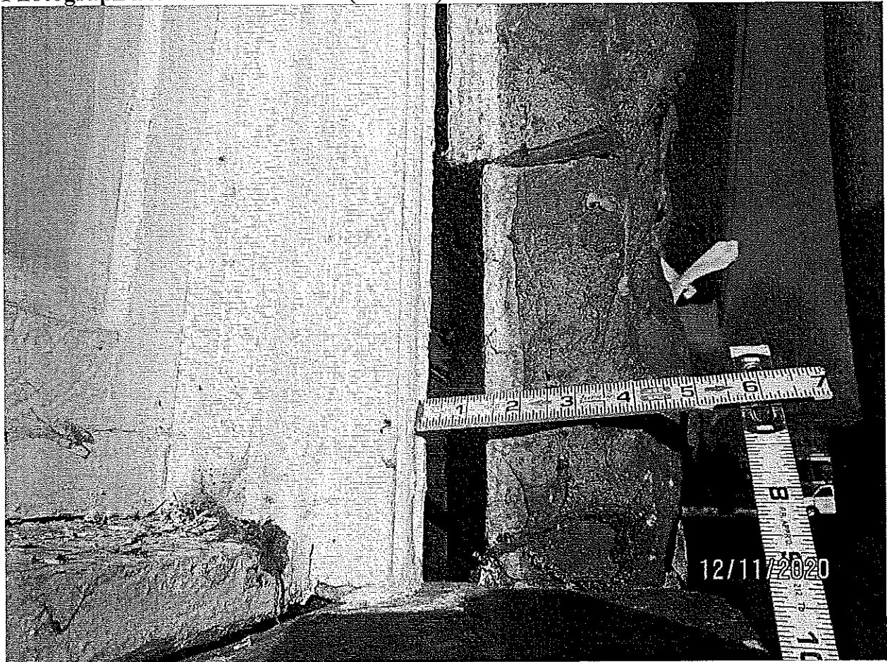
Photograph 24: Wall movement (left side) at window casement.
