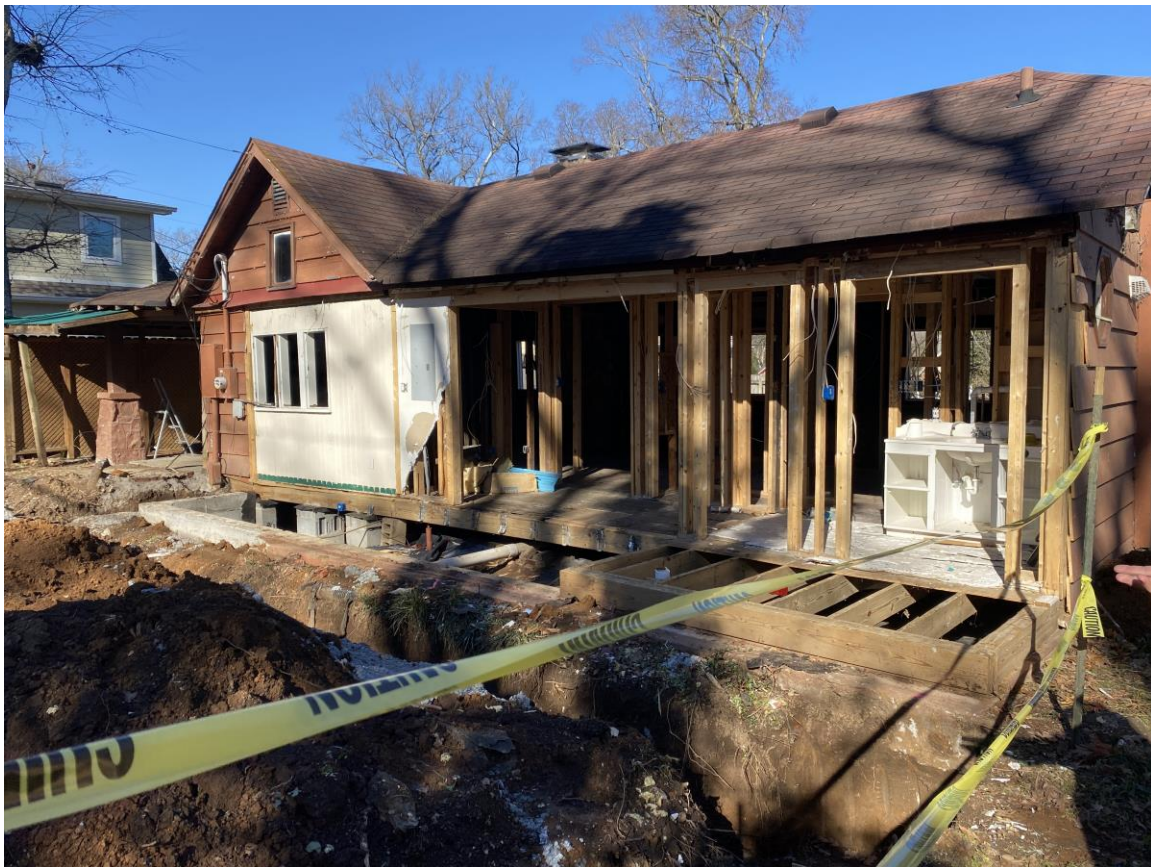
Figure 4: Rear of home in December 2020, after rear wall was removed for demolition.
