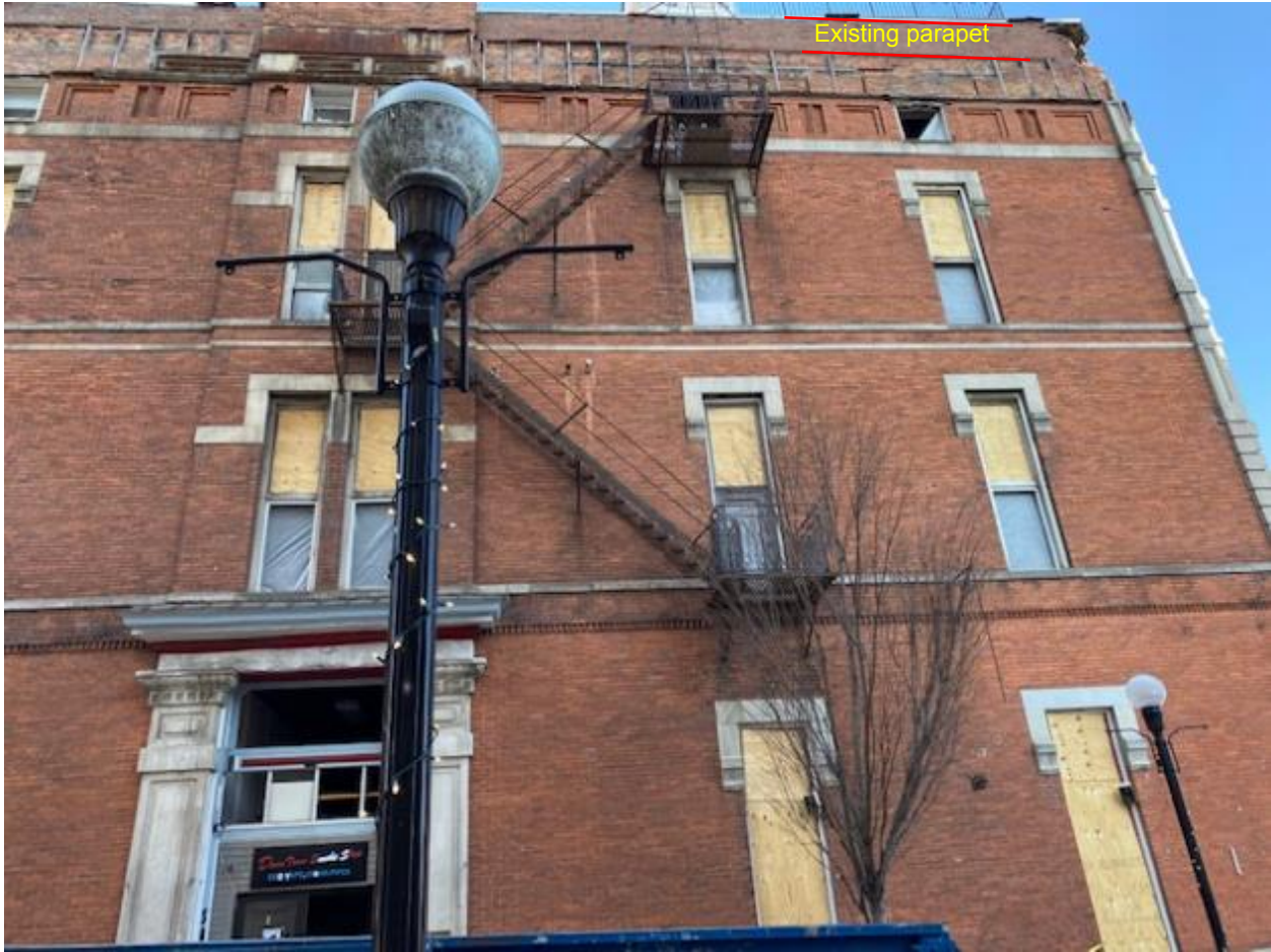
Exhibit 6 Existing parapet and weakened underlying brick, mortar and wood
