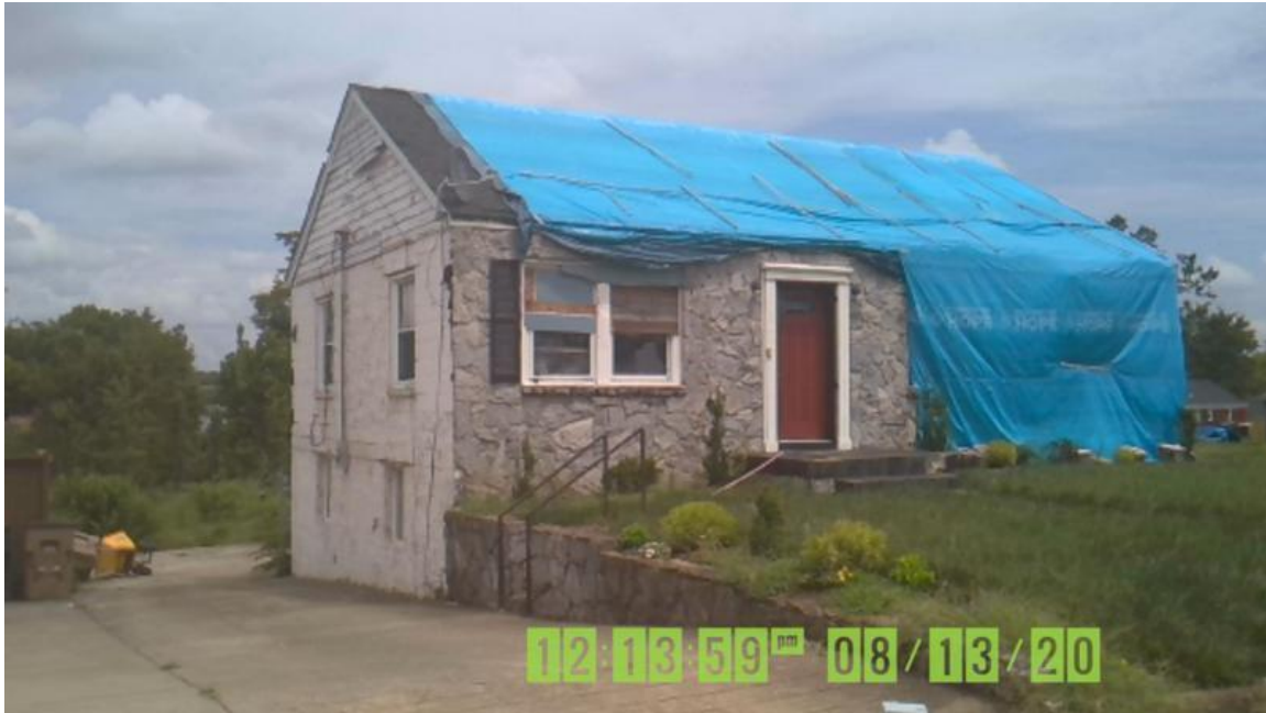
Figure 1. 1809 Holly Street after the March 3, 2020 tornado.
