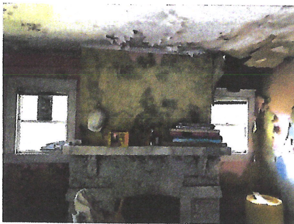
Water Damage – West Wall/Fireplace
