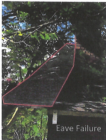
Roof Damage – West Wall/Roof
