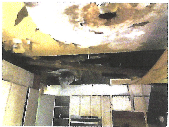
Water Damage – Kitchen Ceiling Collapse
