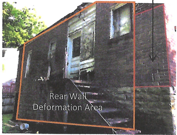
Rear Wall Deformation Area North (Rear) Facade
