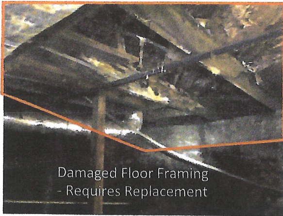
Damaged Floor Framing - Requires Replacement Water Damage – West Wall/Floor Joists
