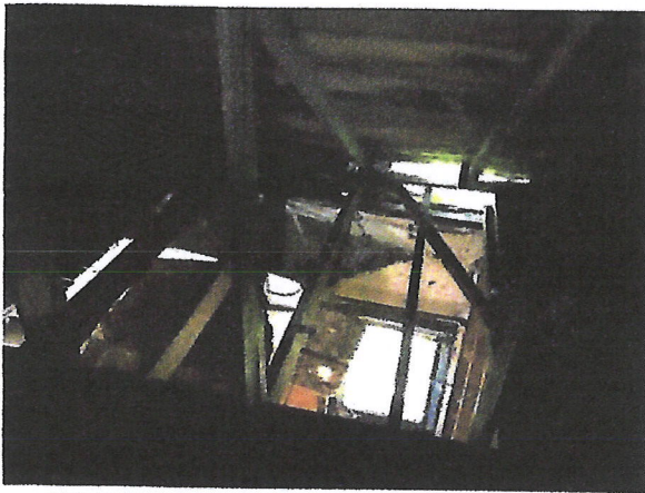
Water Damage – Kitchen Ceiling Collapse
