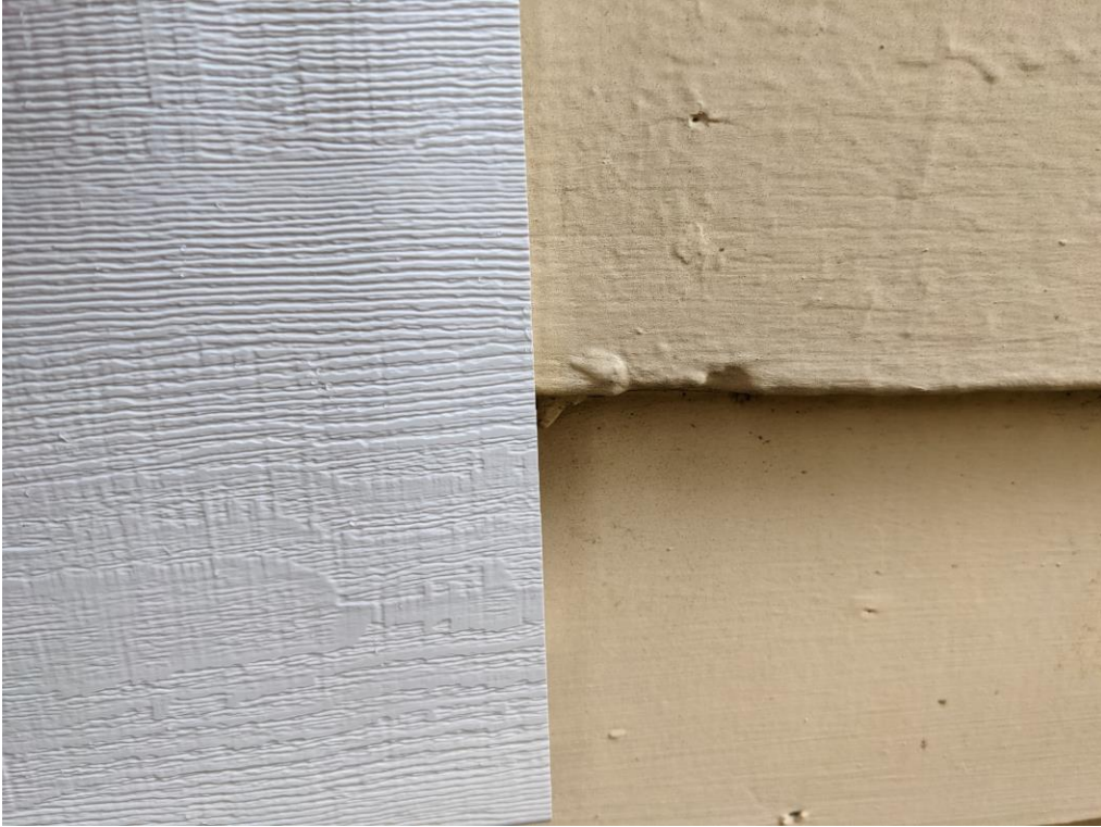
The proposed siding is on the left. Historic siding is seen top, right and replacement wood siding is seen bottom right.
