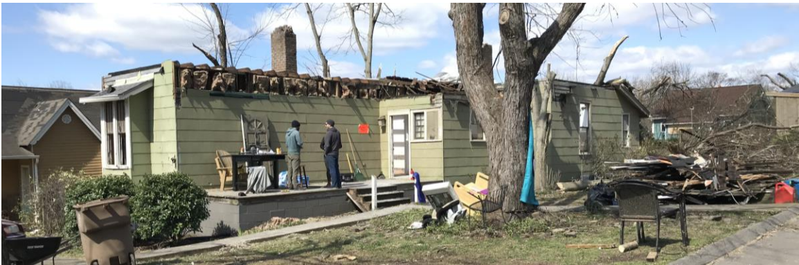
Figure 3. The tornado damage
