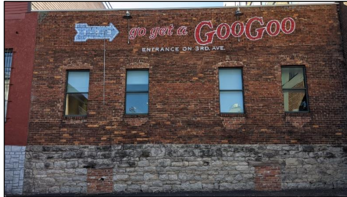
Figure 2: Rear façade of 116 3 rd Avenue South. This wall is to be rebuilt, with a new windows and similar painted sign one hundred, twenty square feet (120 sq. ft.) in size.
