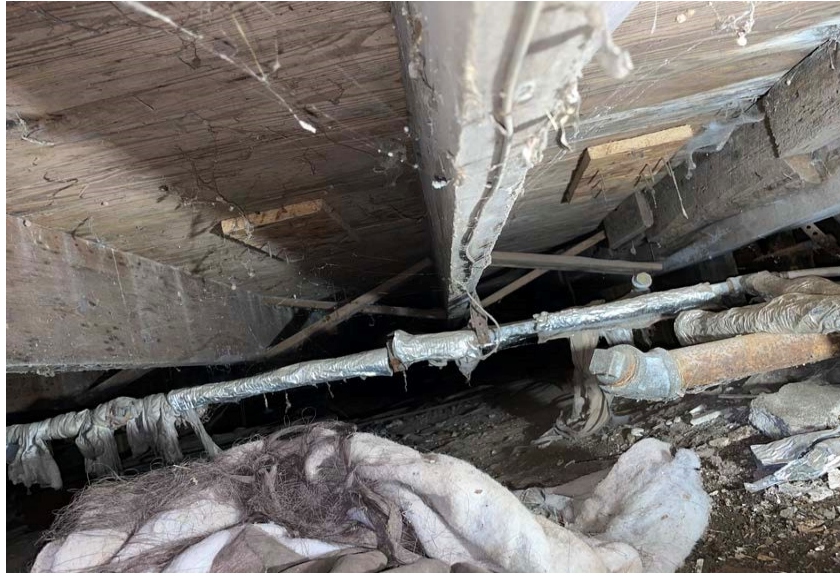
View of Crawl Space – No accessibility; No vapor barrier
