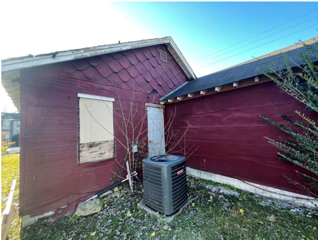
View of East Corner (Rear) of House next to addition (Note: Poor installation of siding – wrinkles and waves)
