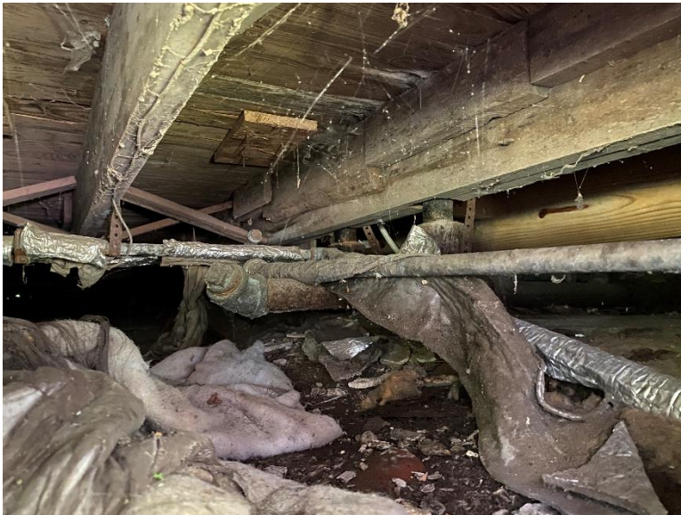
Figure 3. Damaged/deteriorated structural components underneath.
