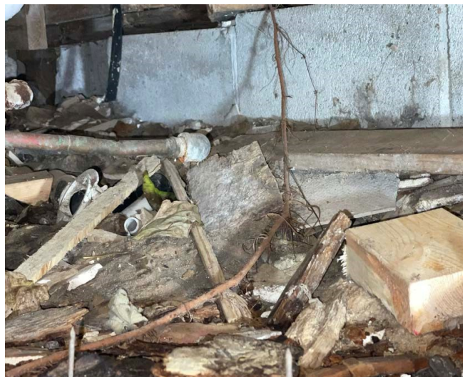
View of Debris in Crawl Space (Note CMU foundation wall)
