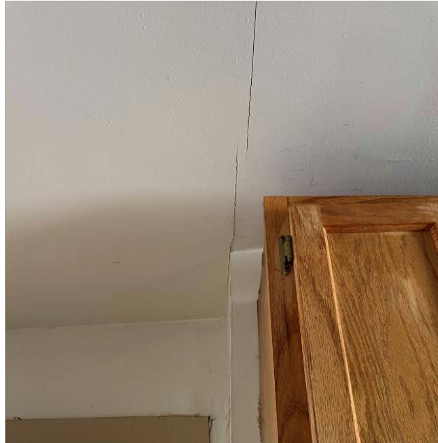
Separation crack in kitchen ceiling
