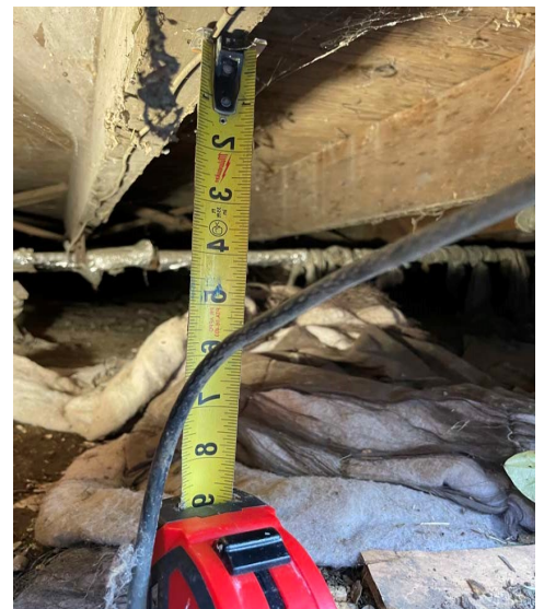
Head Space in Crawl Space Less than 12"
