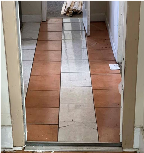
Cracked Uneven Tile Floor
