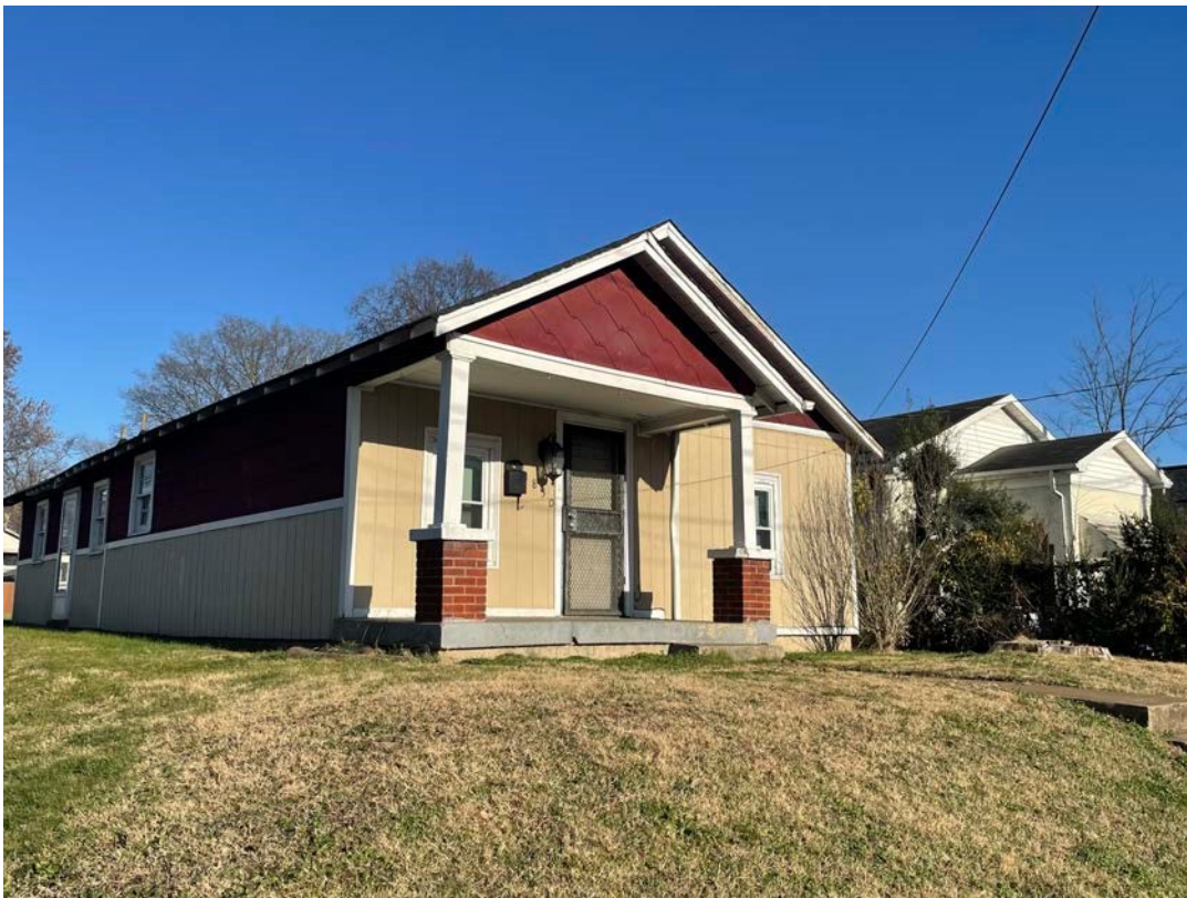
View of Front and North Side (Porch slab is cracked and heaves in middle)
