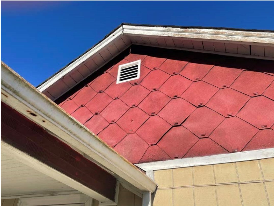
View of somewhat fancy asphalt siding shingles (Note the only gutter on the house on the porch)
