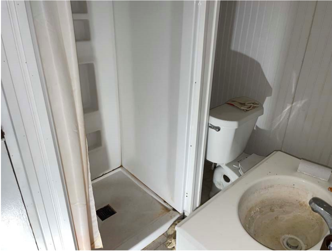
View of Bathroom – Not compliant with codes
