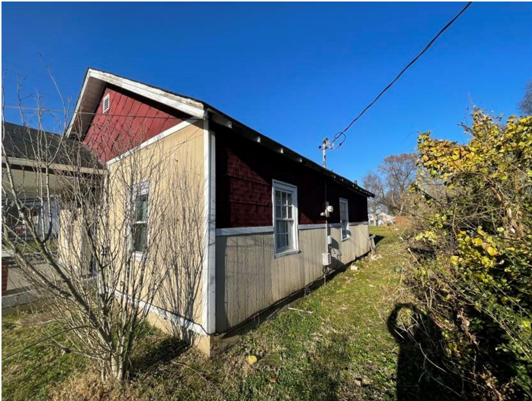
View of South Side from Front Corner (Note poorly attached wood panel siding- wavy;)
