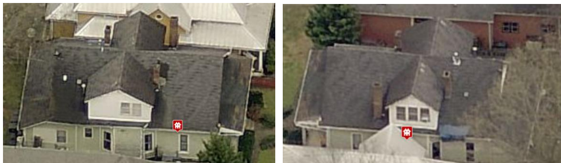
Figure 2 (left) is the left side dormer and Figure 3 (right) is the right side dormer.
