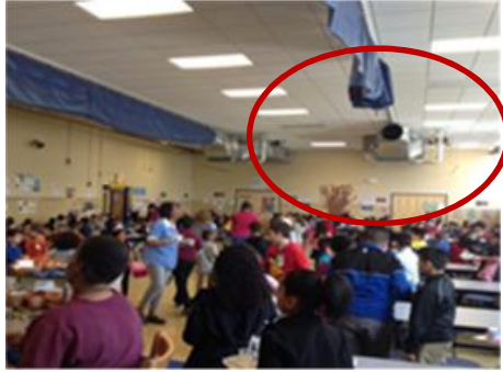
PHOTO #5: Cole Elementary School Duct disconnected from unit
