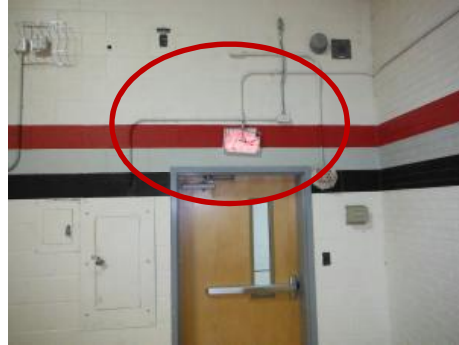
PHOTO #6: Wright Middle School Missing exit sign
