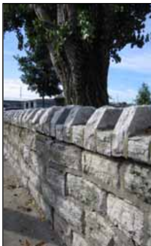
Future tuck-pointing could extend life of perimeter wall
