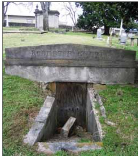
Ground vaults are a unique feature in the cemetery and are in need of structural evaluation
