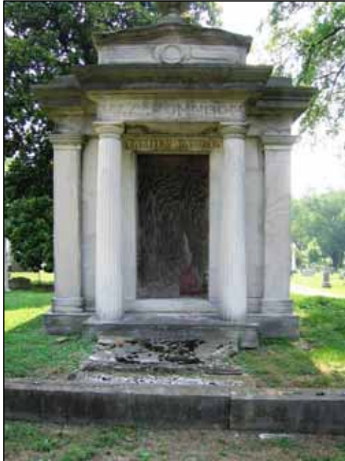
Above: The W.A. Johnson family vault offers a great opportunity for interpretation and as use as a demonstration project. This mausoleum is a fine example of the craftsmanship and artistry available during the Cemetery's period of significance.
