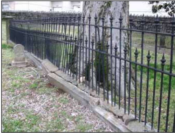
Tree growth causing structural damage
