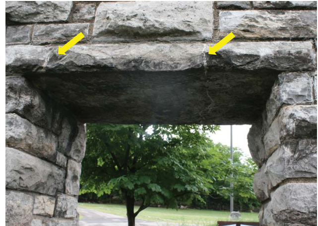
Figure 97. Lintel over wall opening at entrance gate cracked in two places (JMA, 2013).
