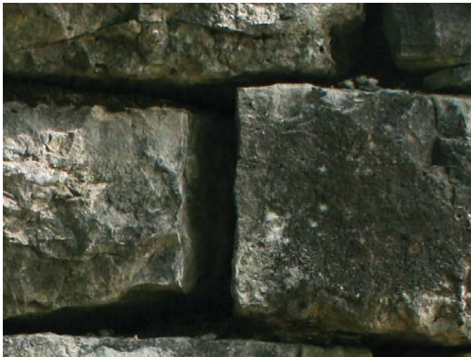
Figure 80. Open head joints (JMA, 2013).
