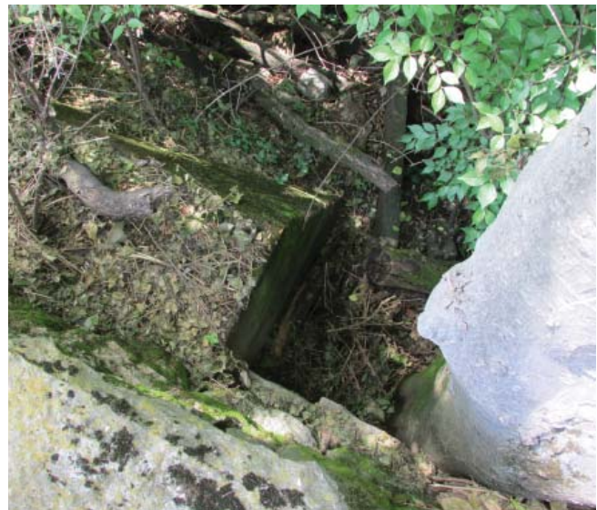
Figure 115. Loss of capstone units and delamination of exterior surface of stones. (1200AE).
