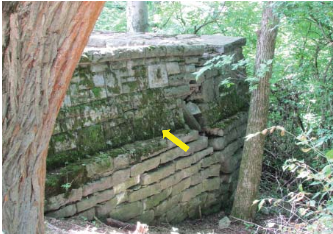
Figure 112. Parapet wall construction on top of dry-stacked stone wall (yellow arrow) and collapse at NW corner of wall due to sliding of corner down the hill (1200AE, 2013).
