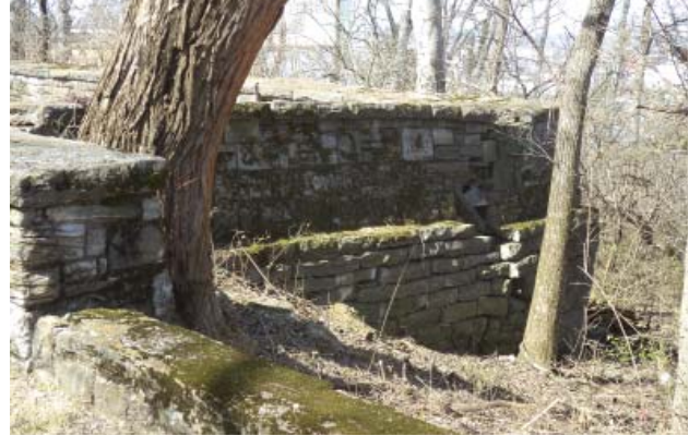
Figure 35. Northeast corner of parking area retaining wall and parapet (JMA, 2013). The loop road wall in the foreground abuts the southeast end of the parking area parapet.
