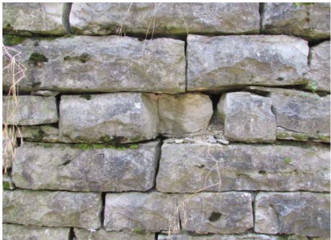
Figure 72. Loss of stone due to spalling and vertical flexural cracks above and below (1200 AE, 2013).
