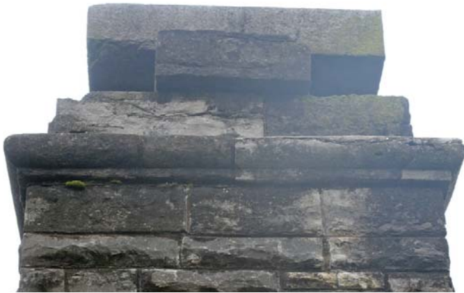
Figure 94. Open joints at top of north pylon at entrance gate with accompanying efflorescence, biological growth including moss, and erosion of natural cracks in two limestone units (JMA, 2013).
