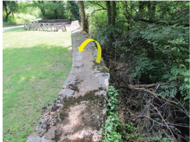
Figure 114. Rotation of parapet towards the interior (1200AE, 2013).
