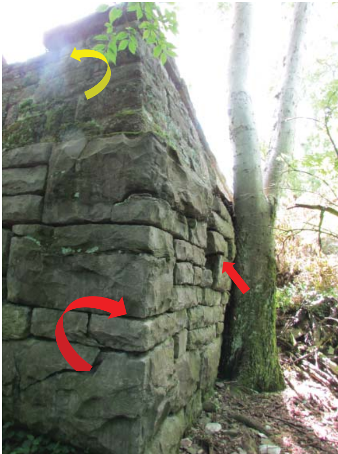
Figure 113. Typical wall conditions at parking area retaining wall. Note bulging and out-of-plane rotation in the dry-stacked retaining wall (red arrows) and out-of-plane rotation of parapet towards interior (yellow arrow). Note position of tree and restricting additional lateral movement. (1200AE, 2013).
