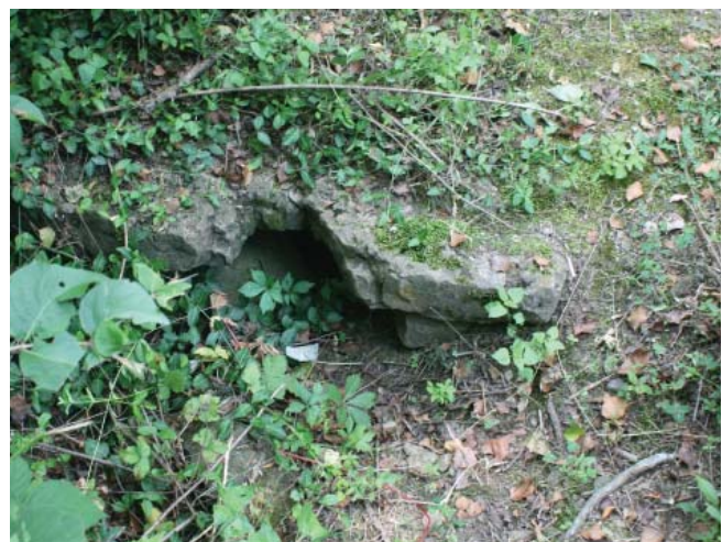
Figure 116. Partially-buried limestone drop inlet cover (JMA, 2013).
