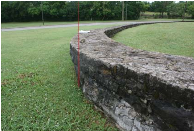
Figure 106. Section of northwest wing wall of entrance gate structure exhibits bowing resulting from either vehicular damage or an underlying structural problem (JMA, 2013).
