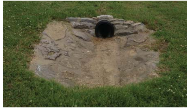
Figure 40. Drainage outlet extending from concrete catch basin inside the loop road (JMA, 2013).
