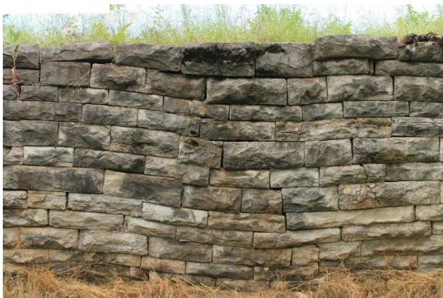
Figure 76. Sagging wall, possibly due to poor soils, animal burrows, or undermining (JMA, 2013).
