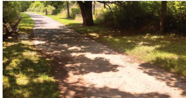
Figure 108. Damp road surfaces at edge indicate locations of ponding (LEA, 2013).
