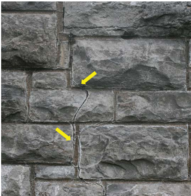
Figure 95. Cracking in east face of north pylon at entrance gate (JMA, 2013).
