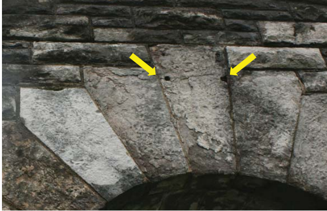
Figure 99. Drilled holes in face of stone in central arch of the entrance gateway (JMA, 2013).
