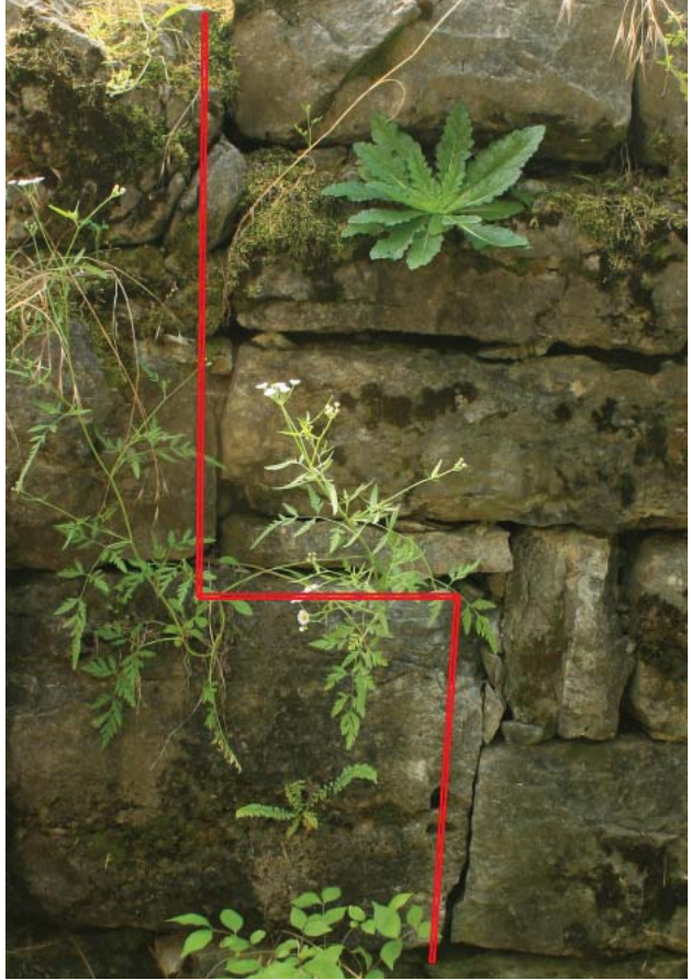
Figure 81. Vertical joints aligned and plant growth in cracks (JMA, 2013).
