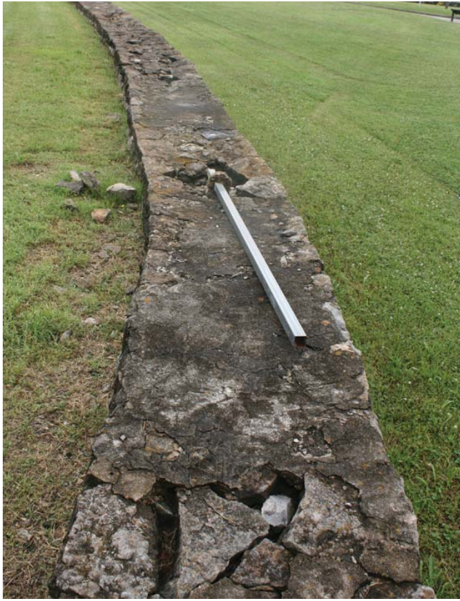
Figure 105. Damage to top surface of northwest wing wall of entrance gate structure caused by water infiltration and failure of post previously mounted into top of wall (JMA, 2013).
