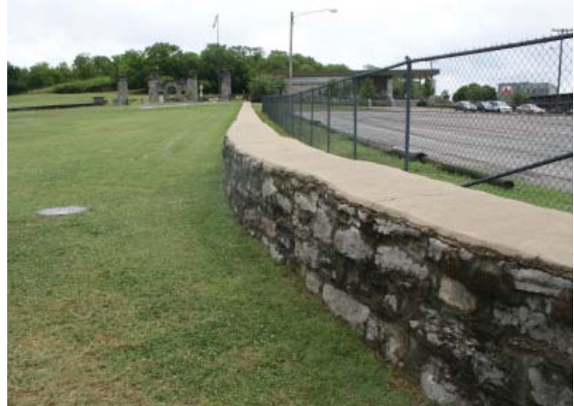
Figure 102. Bowing and displacement of southern wing wall, front view, entrance gate (left) and Visitor Center (right) in background (JMA, 2013).
