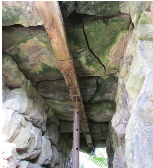
Figure 92. West Bastion tunnel with shoring installed and loss of post shores (1200AE, 2013).
