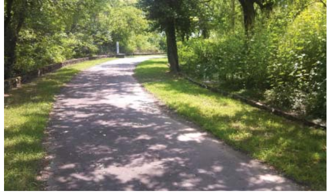
Figure 107. Flat profile of loop road allows water to stand (ponding) after heavy rain (LEA, 2013).
