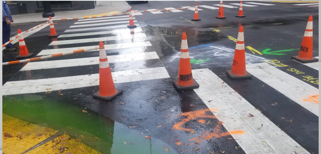
Leak at 4 th and Union
