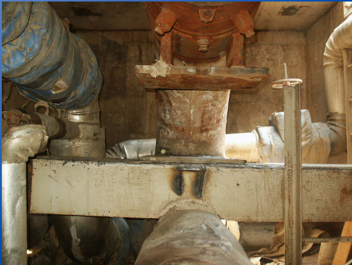
MH-L Piping & Slip Joint
