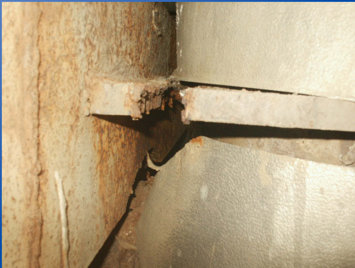
Anchor Plate Failure in MH-L
