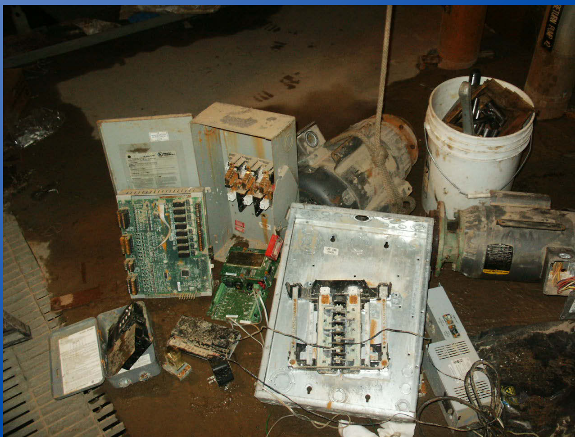
Condensate Pumps in MH-18
